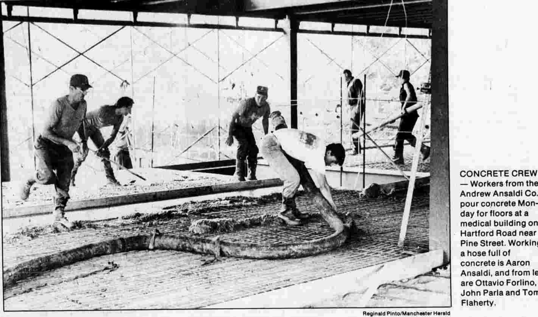
Concrete crew — Workers from the Andrew Ansaldo Co. pour concrete Monday for floors at a medical building on Hartford Road near Pine Street, Working a hose full of concrete is Aaron Ansaldo, and from left are Ottavio Forlino, John Parla and Tom Flaherty.
