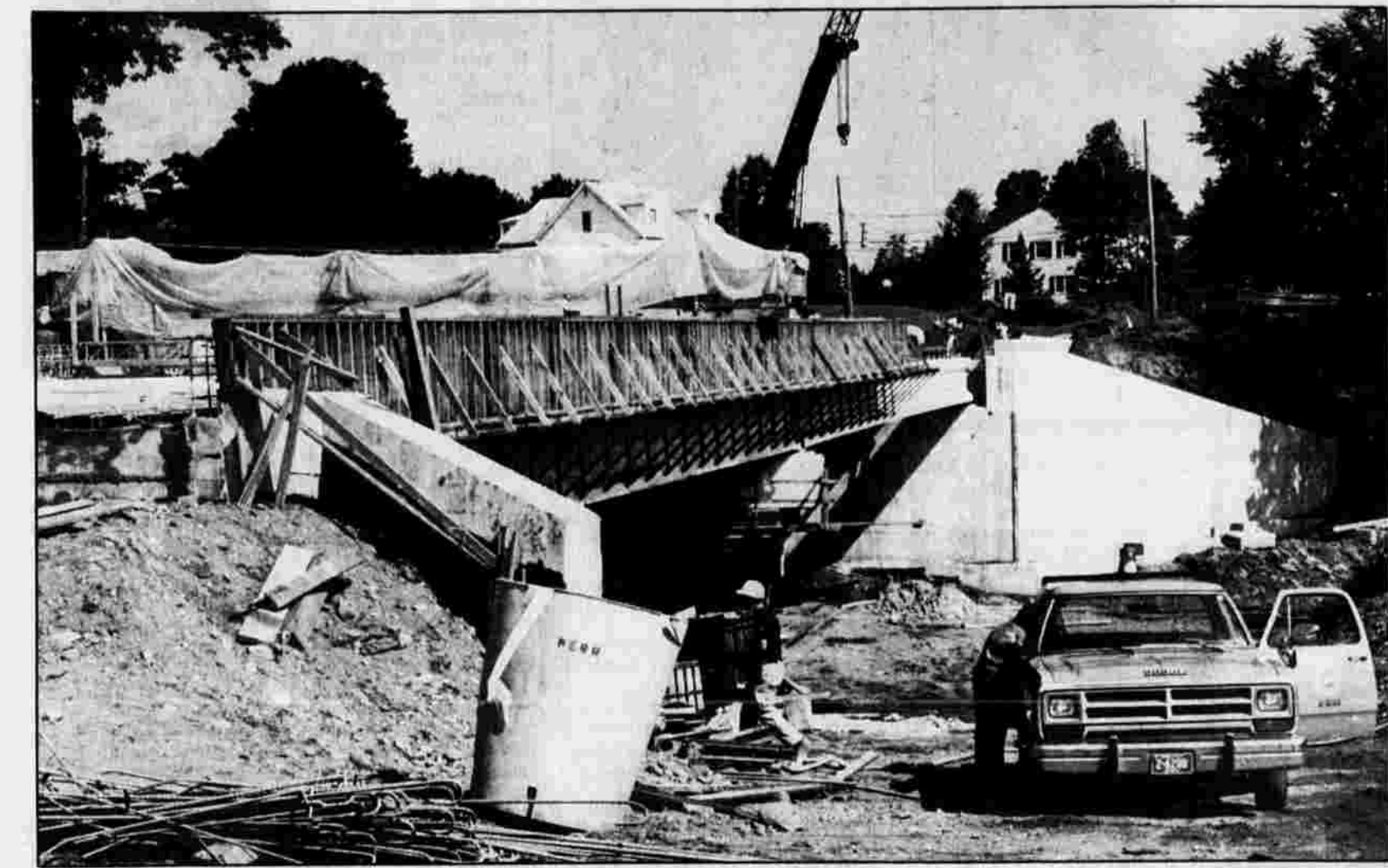
BRIDGING THE GAP — A crane hovers above the Union Street construction project Monday. The new bridge is being built on the east side of the existing bridge. The
